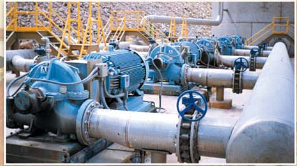
All 316 stainless steel model 3409 pumps on a solvent extraction application at a large copper mine.
