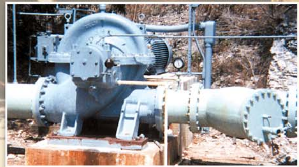
Model 3420 splitcase pump in service at an electric utility plant in the Bahamas.
