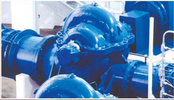
Model 3498 pumping drinking water through a distribution network in the Western United States.
